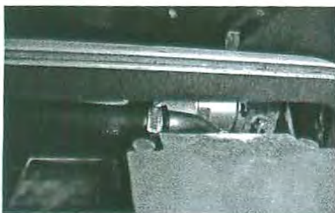
Heat exchanger in normal configuration (Outboard forward corner viewed from above)
