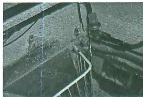
Expansion valve in freezer
