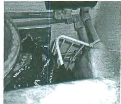
Second holding plate showing large and small pipe sets
