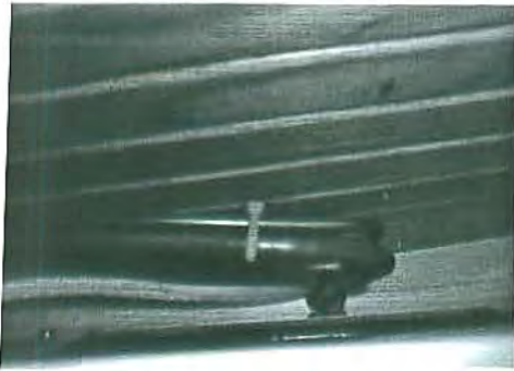
Pipes and power coming up through the counter top
