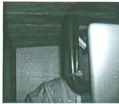
Pipes and power going into the unit
