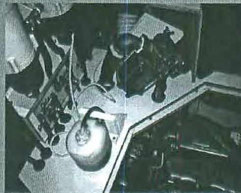
Access to Yanmar seawater anti-siphon valve.
